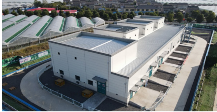
Fig. 3. Real scene of a 110kV substation
